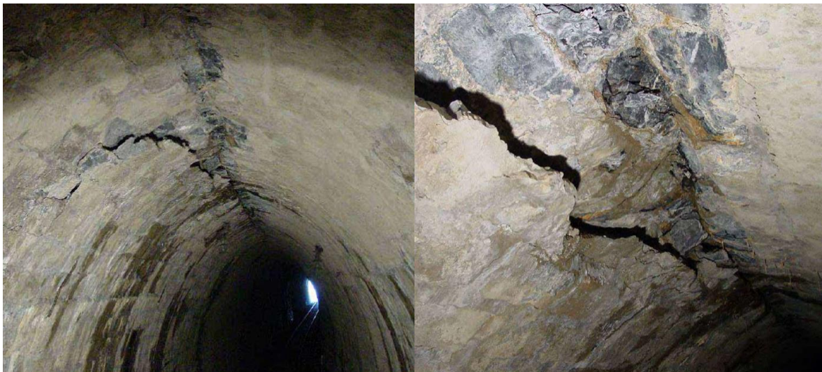
Figure II.14. Fissures en sifflet
