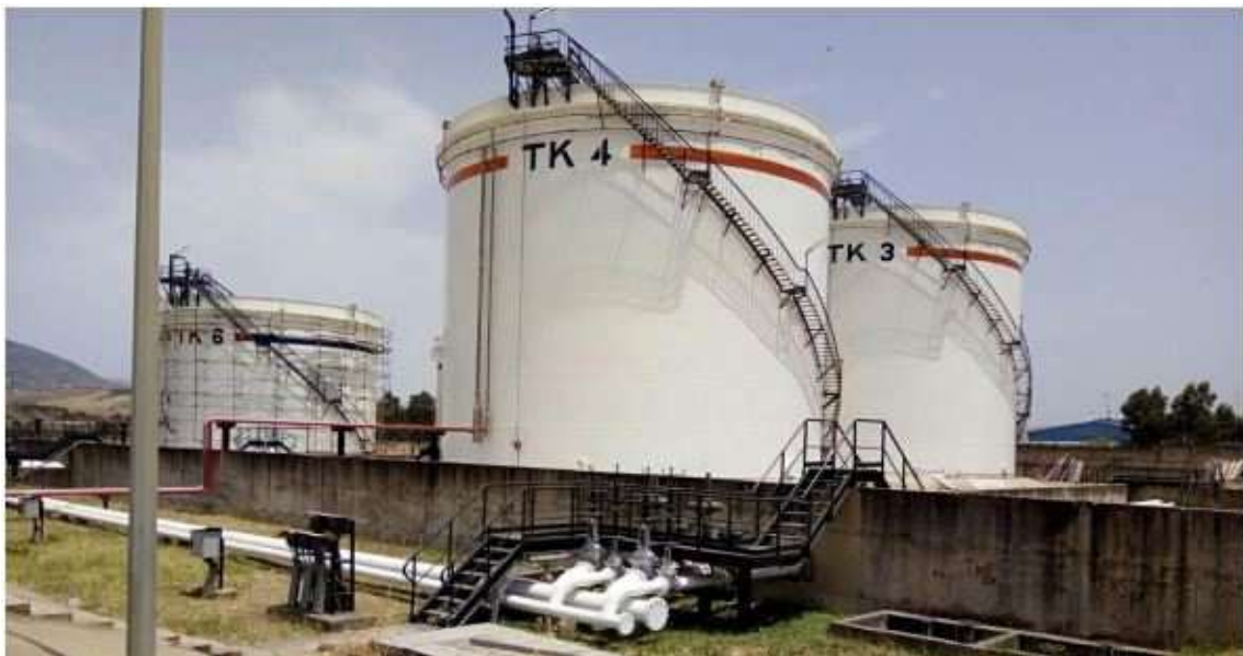
Figure I-3 : bacs de stockage (2)
