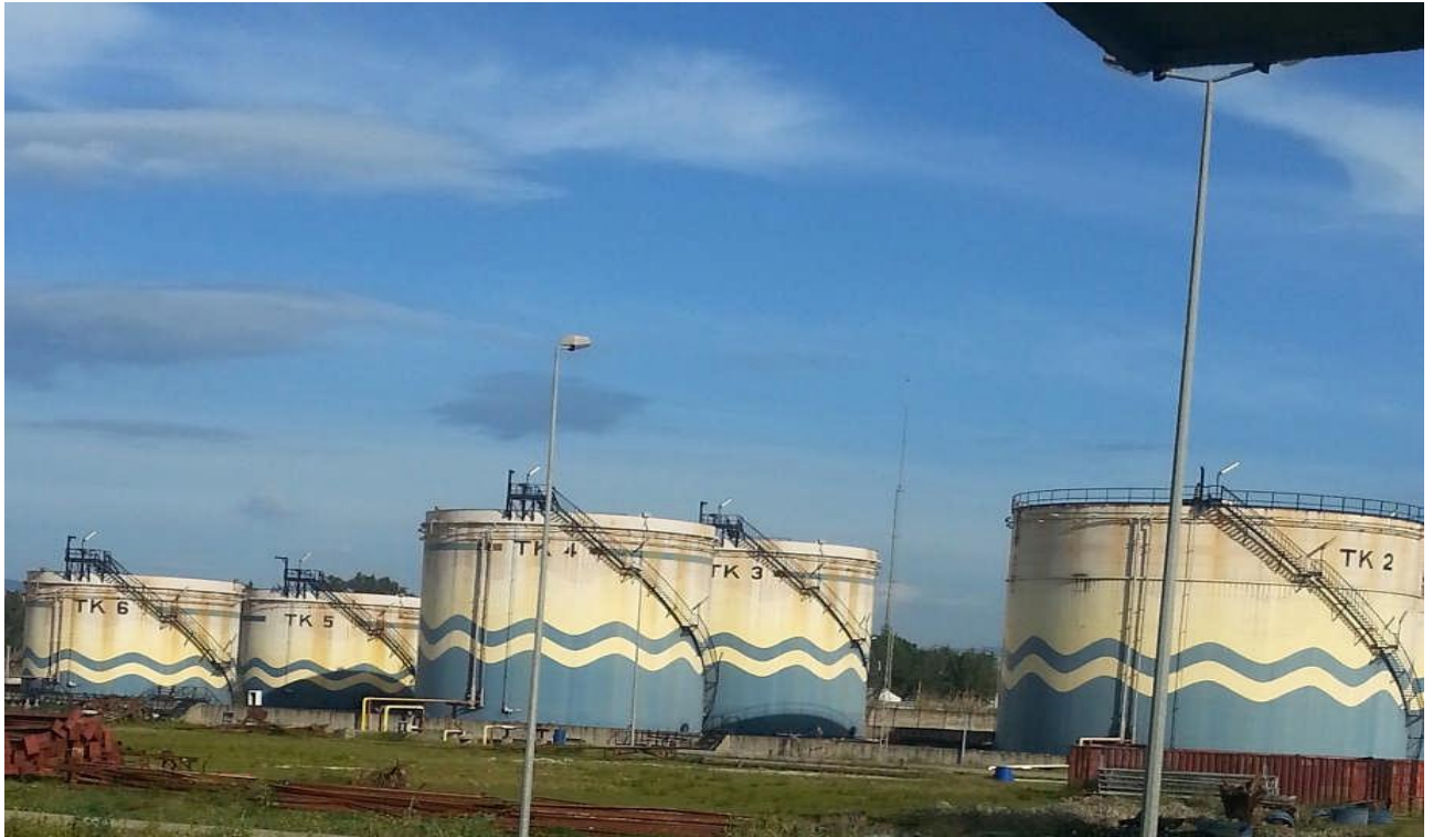
Figure I.2 bacs de stockage.
