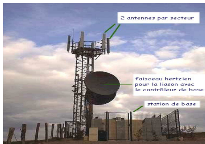
Figure 1 : Station de base
