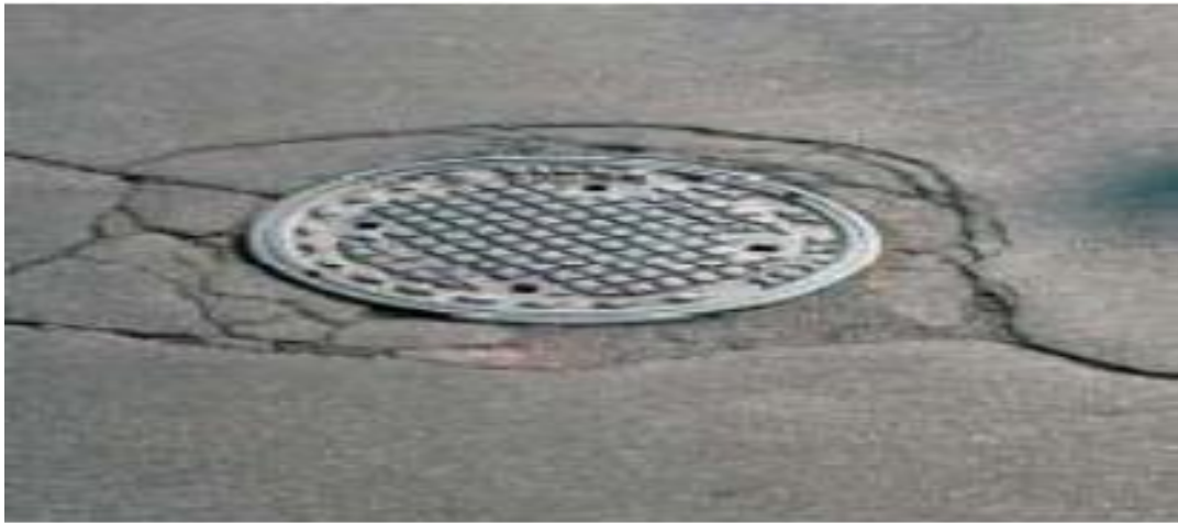
Figure 2.19. Fissuration autour des regards
