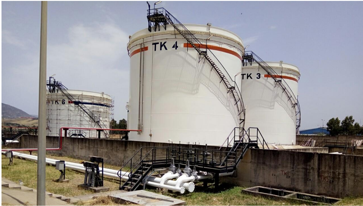
Figure I.3: Le bac de stockage.
