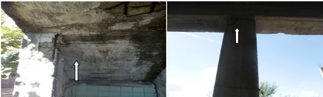
Fig. II.11 : Fissuration des poteaux
