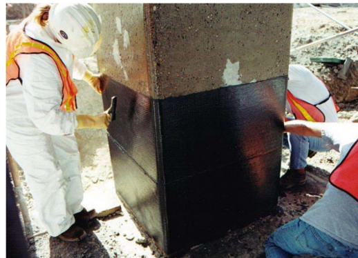
Figure II.23. Confinement de colonnes.
