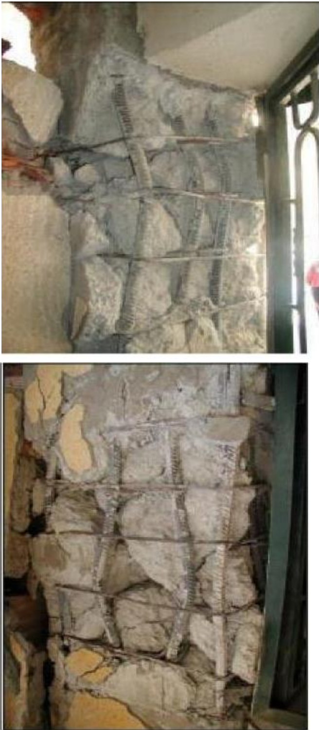
Figure IV.20. Crushing of concrete and buckling of steel in the two posts of the stairwell [10]
