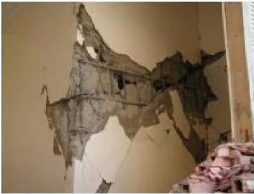
Figure IV.25. Open cracks in the veil [10]
