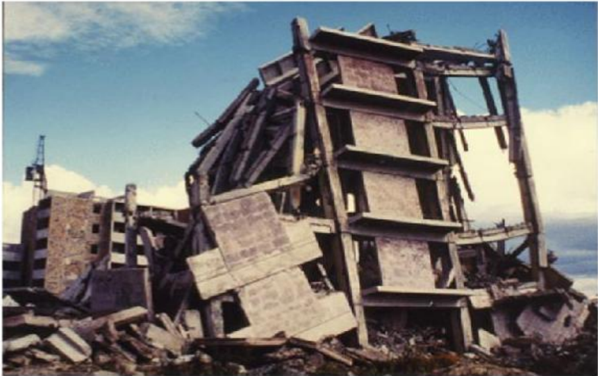
Figure IV.34. Example of very severe structural damage and almost complete collapse.
