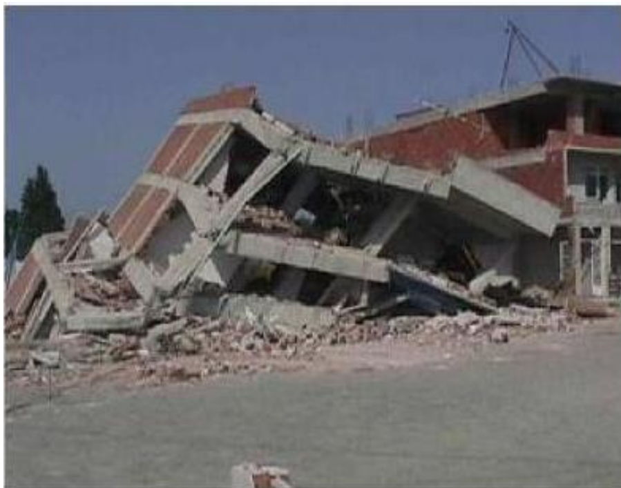
Figure IV.22. Failure by bending of beams [10].
