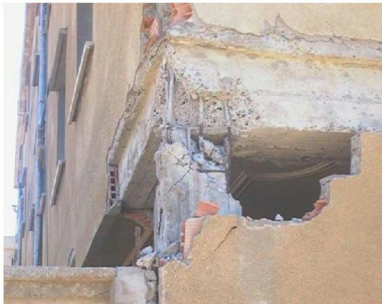
Figure IV.32. Formation of plastic hinge 2003 earthquake, Boumerdes, Algeria
