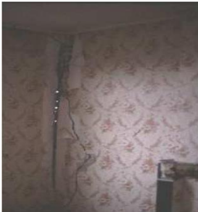
Figure V.17. Liège, 1983. Effect of the weakness of the diaphragms (cracking at the corner of the walls) or the weakness of their connections to the walls (facade collapse)
