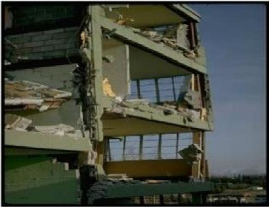
Figure IV.23. Dislocation of masonry fillings [10]
