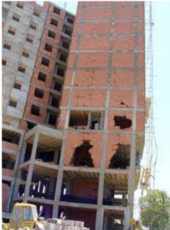
Figure V. 11. Good behavior of a building in nayou (primary structure) and peripheral structure (secondary structure). (Boumerdes, 2003)
