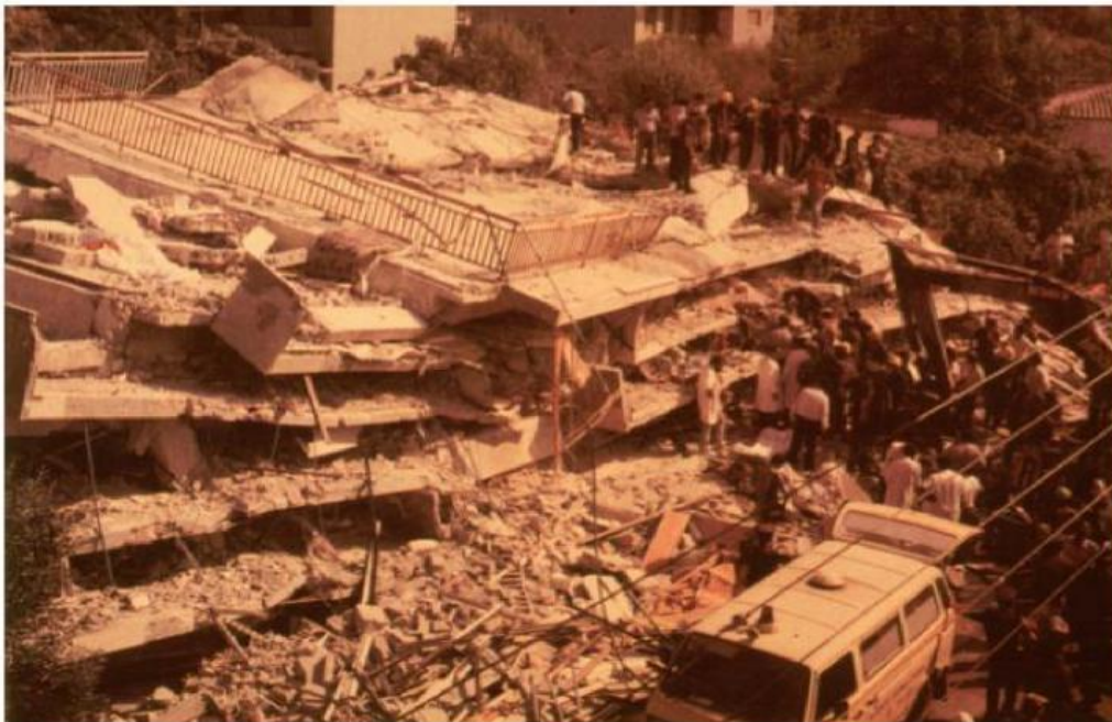
Figure.IV.28. Total collapse of unbraced or poorly braced constructions
