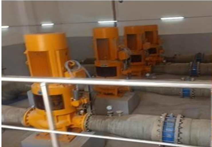
Figure II.6 : Station de relevage (B.N, A.M 2025).
