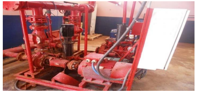
Station de pompes anti-incendie
