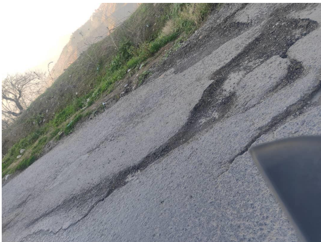
Figure 57 : photo montrant un escarpement de la route du village Ath Sidi Said.
