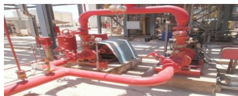
Station des pompes anti-incendie
