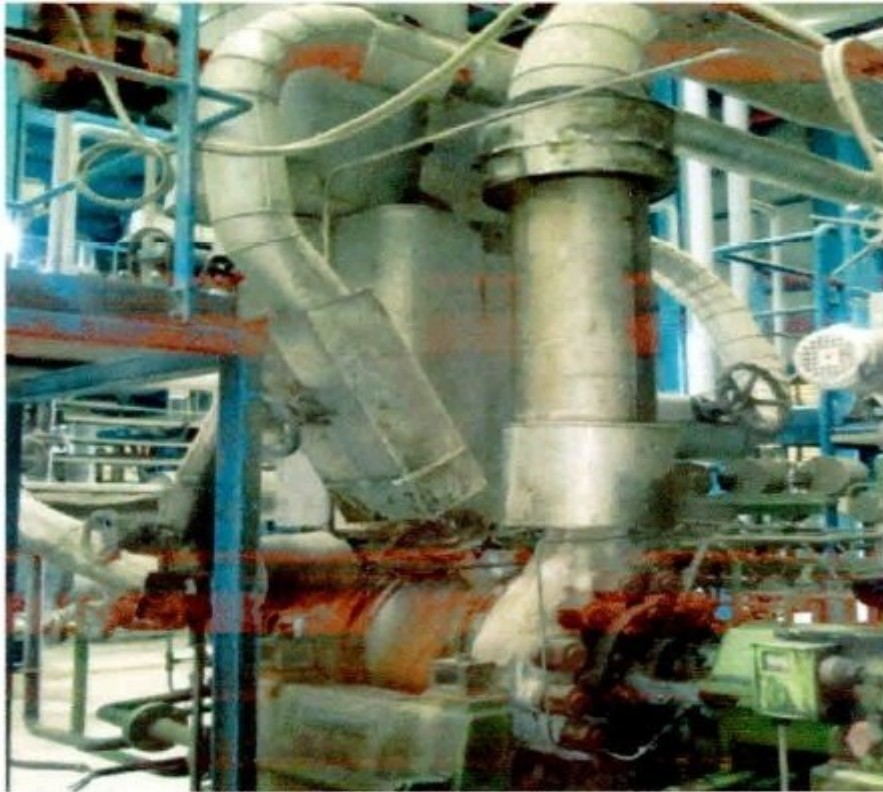
Figure II.5 : Photo de la pompe principale.
