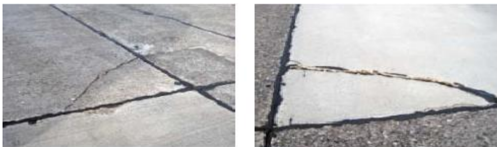
Figure 22 : fissure en coin [5]
